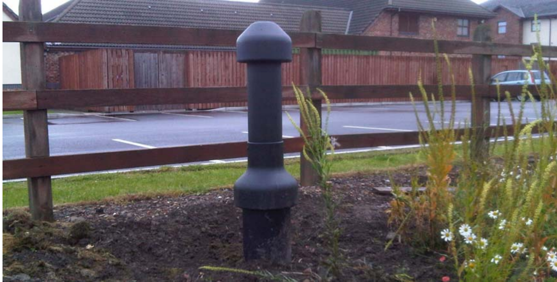
Combination bollard on a virtual curtain gas migration barrier
